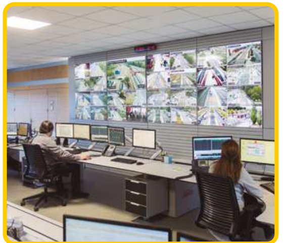
CCC – Central Control Centre
